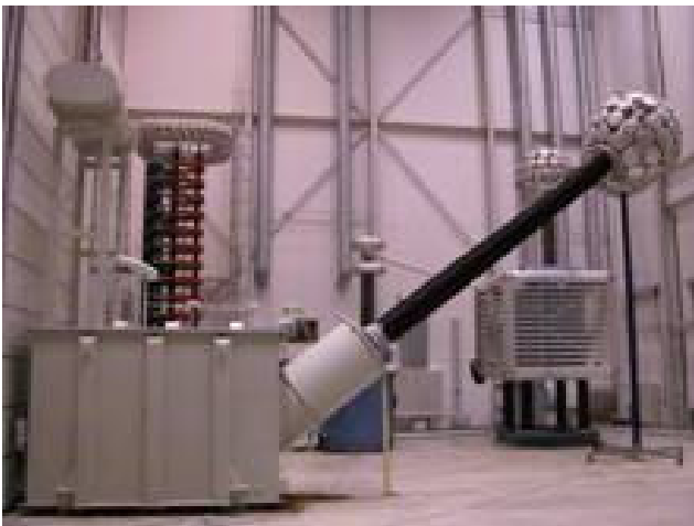
Figure 2: Transformer prototype in test room
