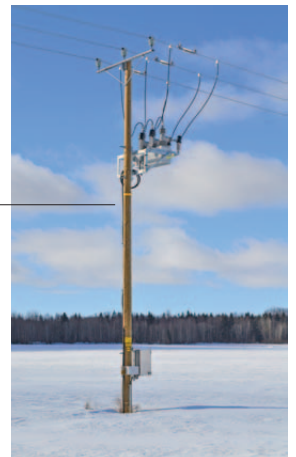
Pole mounted recloser
