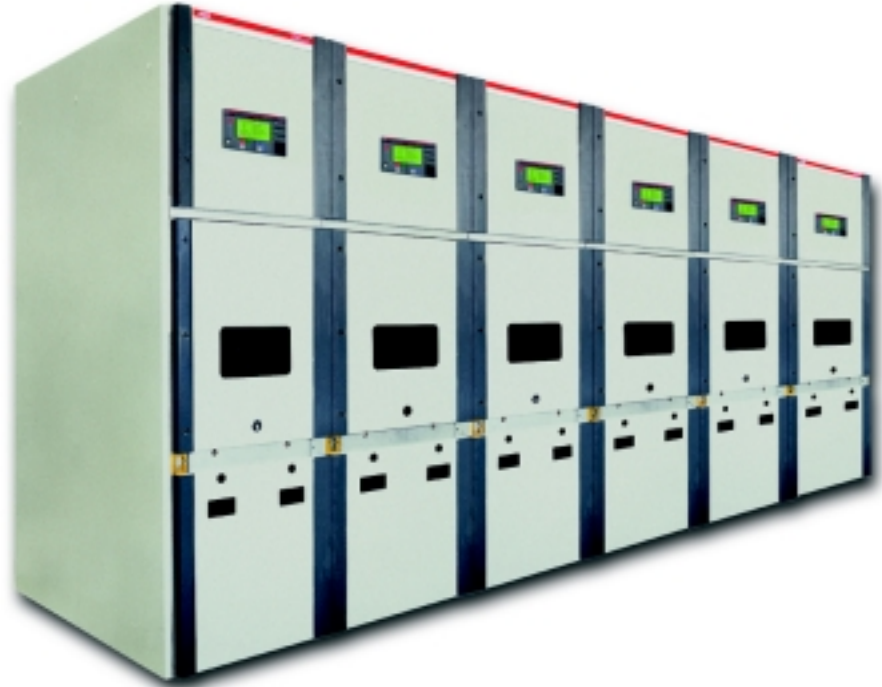
Figure 5: REF542 plus installed in air-insulated switchgears (AIS)
