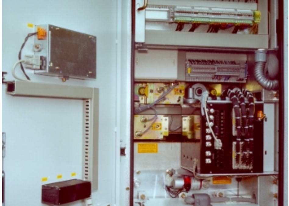
Figure 6: Example of mounting of the Central Unit in the LV compartment and the HMI on the door
