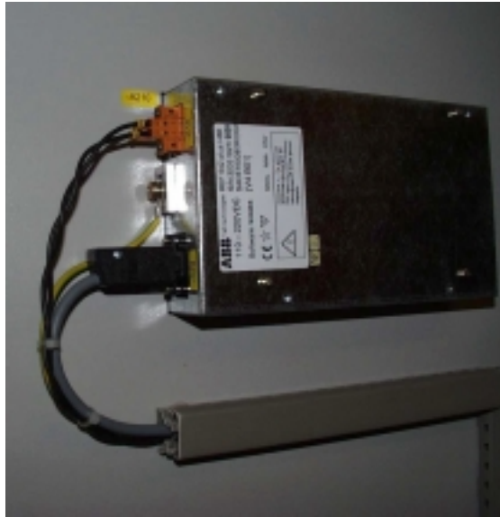
Figure 5: Grounding of the REF542 plus HMI Local Control Unit
