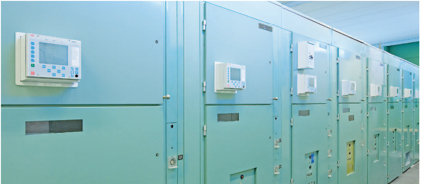
The 630 series IEDs and REA arc protection system were installed in the MEKA 24 switchgear.
