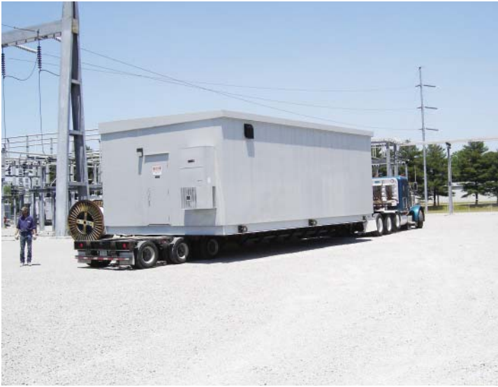
Modular protection and control buildings
