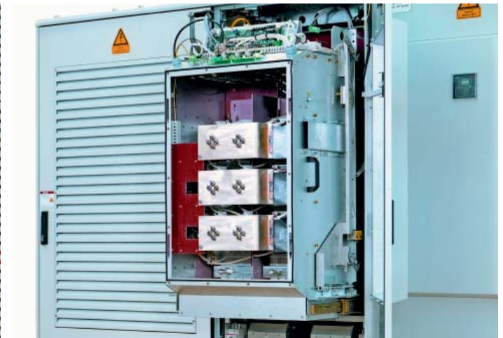
UNL 14300 power converter in draw out position
