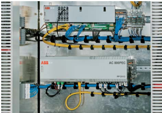
Measuring unit and main control channel of UNITROL 6800
