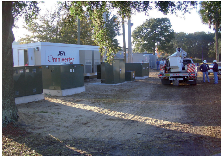
The 2000kVA 26KV PCS100 AVC in its dedicated container on-site
