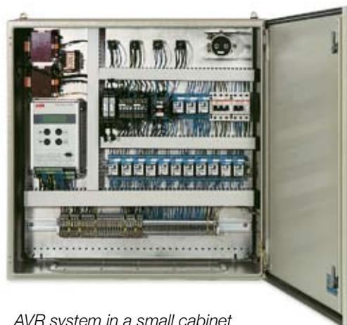
AVR system in a small cabinet
