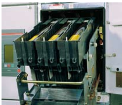
Contactors in the withdrawn position for the fuses control and replacement.
