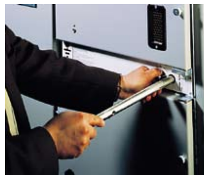
Contactors racking-in with the door closed.
