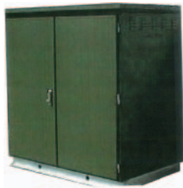
Outdoor Motor Control Centre
