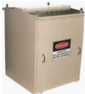
Outdoor Metering Cubicle
