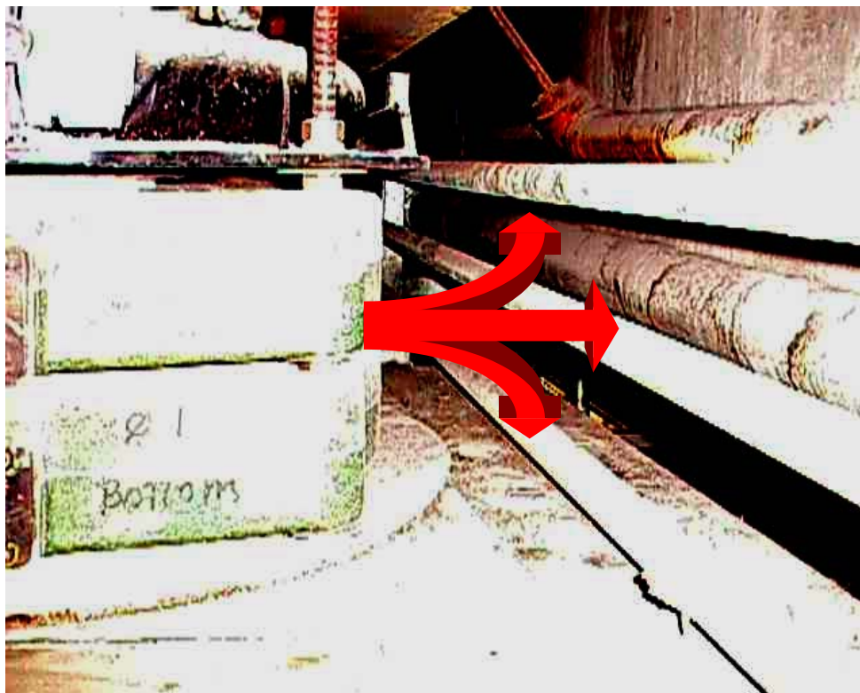
Figure 3. Conduit runs near generator bushing in high magnetic field area
