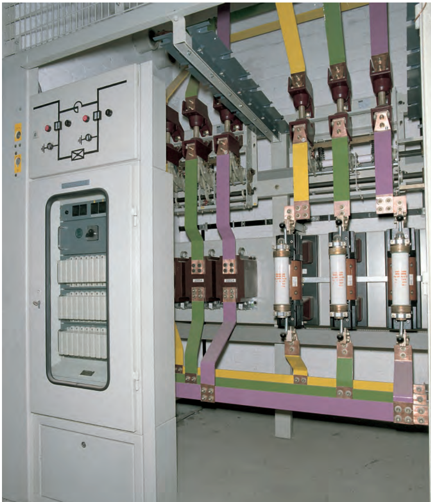
I_s -limiter connected in parallel with a reactor – fixed mounted –
