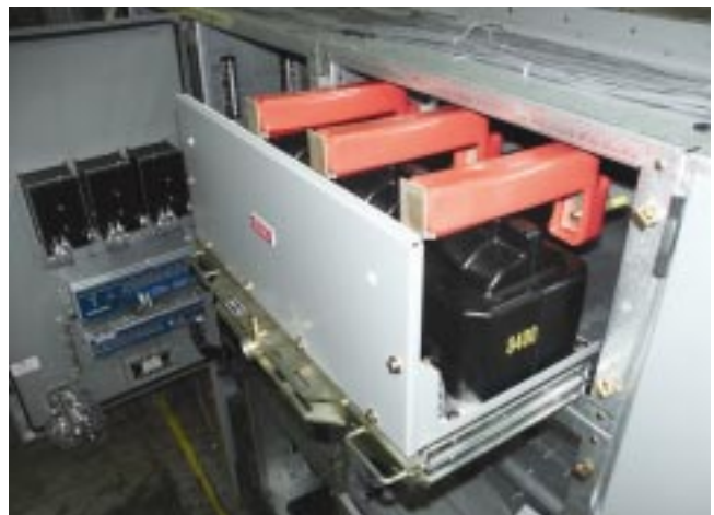
The fuses can be removed without removing the VT truck from the rails.
