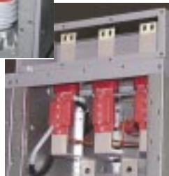
Bus risers to bus duct or roof busings
