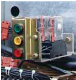
SF6 control device with 3 LEDs.
