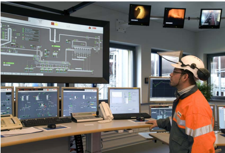
Figure6: ABB control system, Expert Optimizer and Knowledge Manager are installed at the Jura Cement Plant, Switzerland
