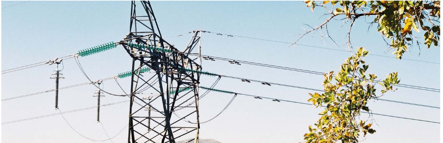
Transmission line arresters, including line discharge class 3 PEXLIM Q arresters and disconnecting devices on earth leads, erected on ESKOM 300 kV system in South Africa.
