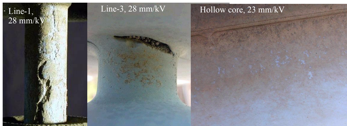
Figure 4 Kelso. Deterioration: comparison of line and hollow insulators.
