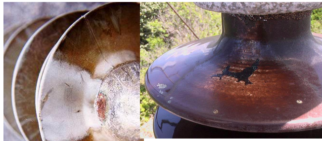
Figure 13 Kelso. Examples of line insulators flashed over due to pollution.
