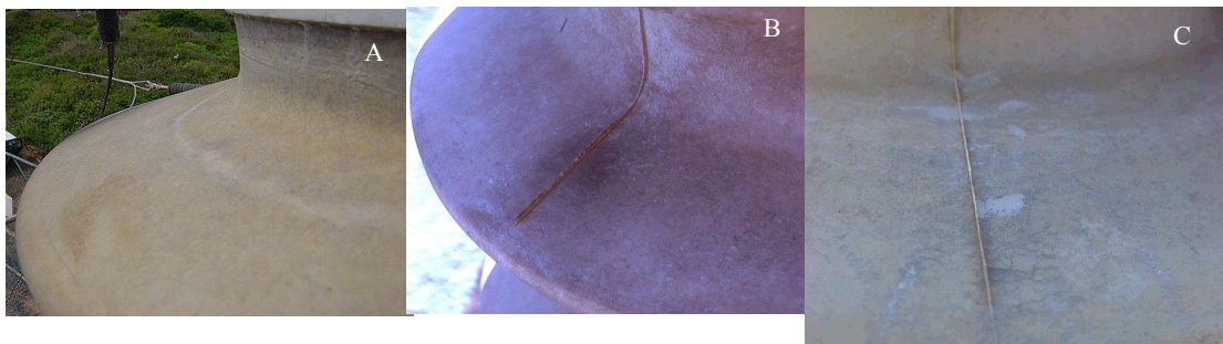
Figure 2 Kelso, apparatus insulators. Examples of deterioration: A: bushing-23, whitish rings; B: arrester-12, dark pattern; C: arrester-16, traces of discharge activity.
