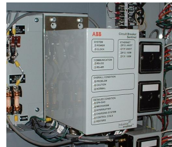
Figure 2 – Circuit Breaker Sentinel
