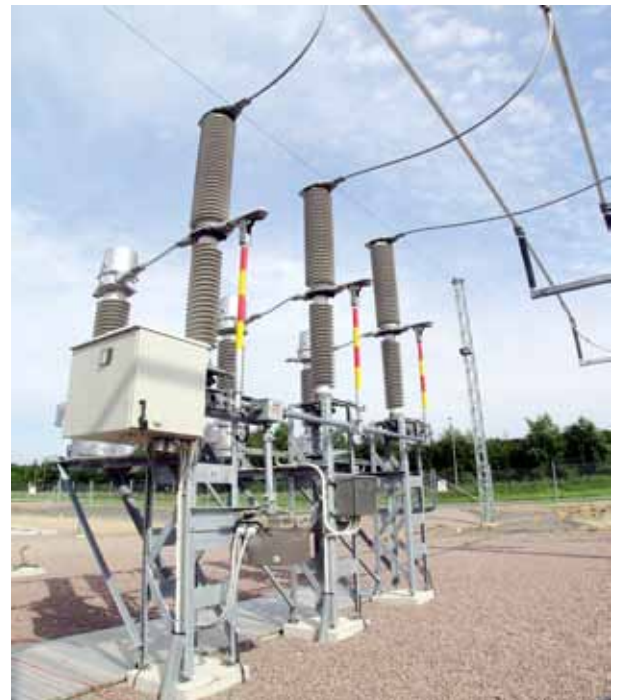
Fig 2. 145 kV DCB with built on current transformers and closed earthing switch
