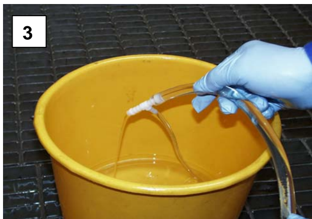
3 Put the hose and T-piece in a bucket. Open the transformer valve. Draw off at least three times the volume of the valve and the hose. Let the oil flow during sam-
