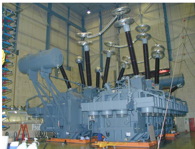
The phase shifters with TEC, tap-changers and bushings from Components.
