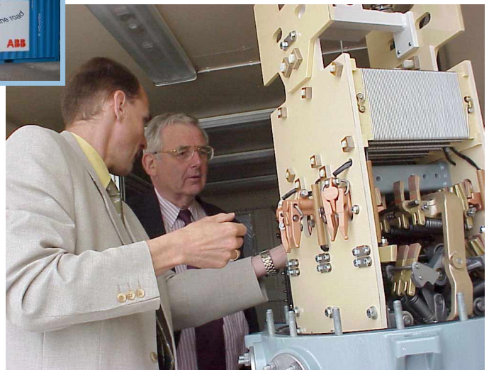
Inside the container at GPU PowerNet in Walsall. Lars Lidén with Mr Barry Lowe, Procurement Manager.
