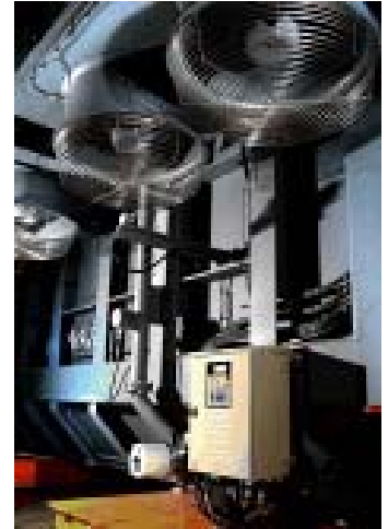
The Terna transformer is equipped with the TrafoStar Electronic Control system.
