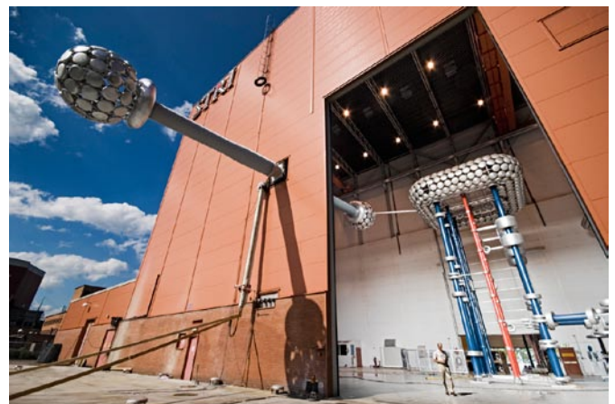
Testing of the first 800 kV dc wall bushing at STRI, Ludvika, Sweden
