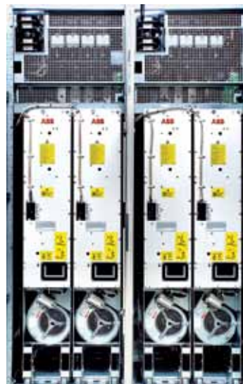
ABB industrial drive modules installed into SAMI STAR drive cabinets in a retrofit.
