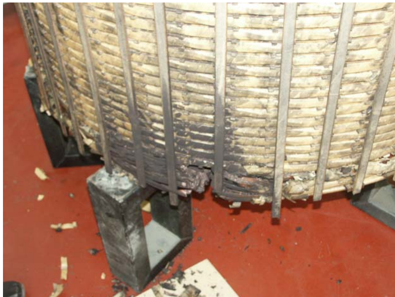
Figure 13. Turn-to-turn fault at the end of the common winding of the Autotransformer Tr3 (Courtesy of Croatian Utility – HEP)
